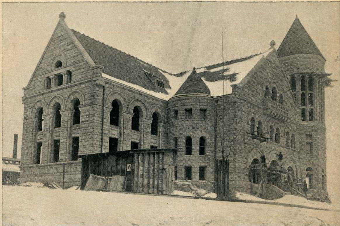
NEW LIBRARY. WEST VIRGINIA UNIVERSITY, IN PROCESS OF CONSTRUCTION; COST OF BUILDING $105,000.
